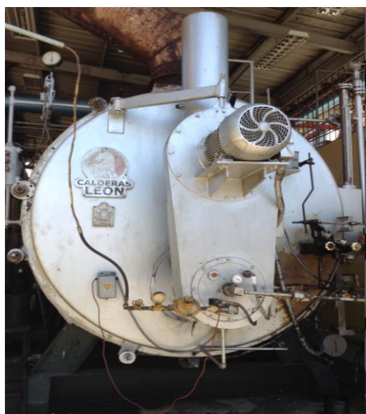
Figure 2. Image of the boiler used
